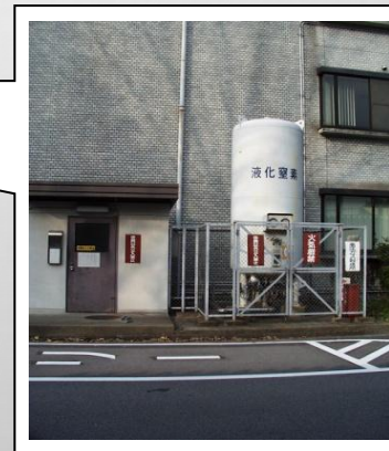
Liquid Nitrogen Dispensing Shed
