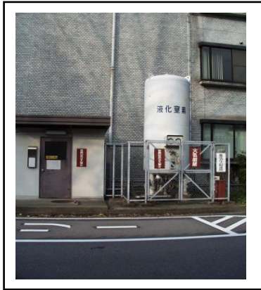
Liquid nitrogen supply point (East side of CACS Office)
